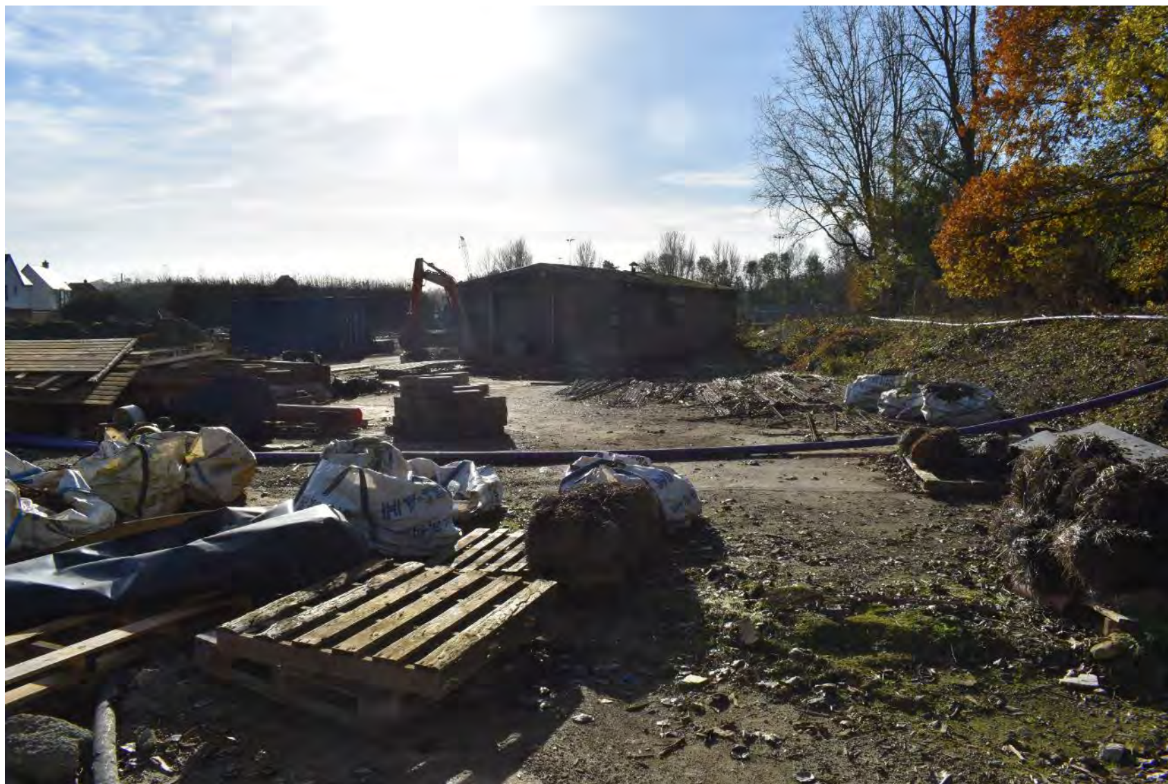
Plate 17: View of part the eastern side of the main area (facing SSW)
