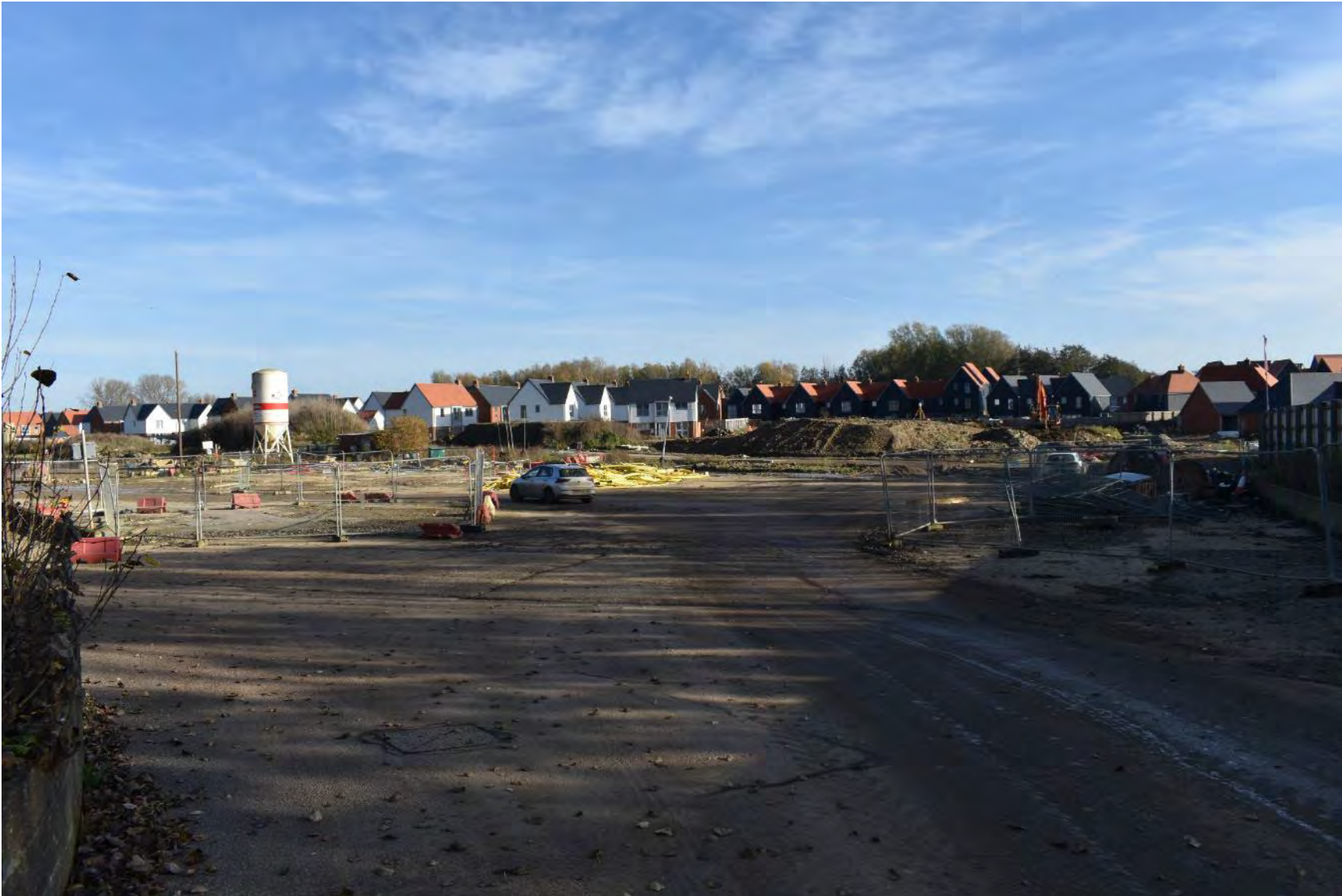
Plate 21: View across the southern end of the western part of the main Application Site (facing E)
